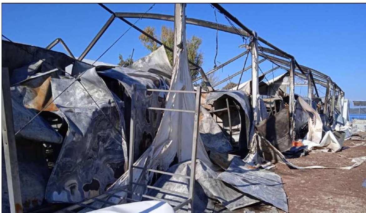
The remaining metallic structure of a rubhall of the Lesvos RIC after the fires of November 2021, Picture by a camp resident.
